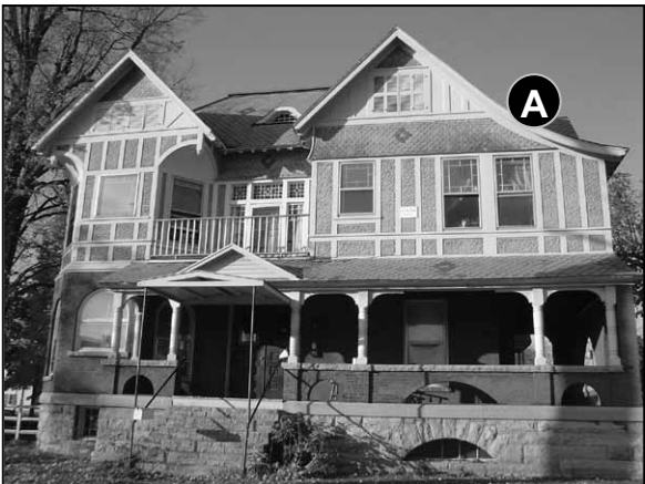
Fig. 5-76: 12 Pleasant St. Paint colors are used here to highlight the different facade materials in this Tudor style house.
