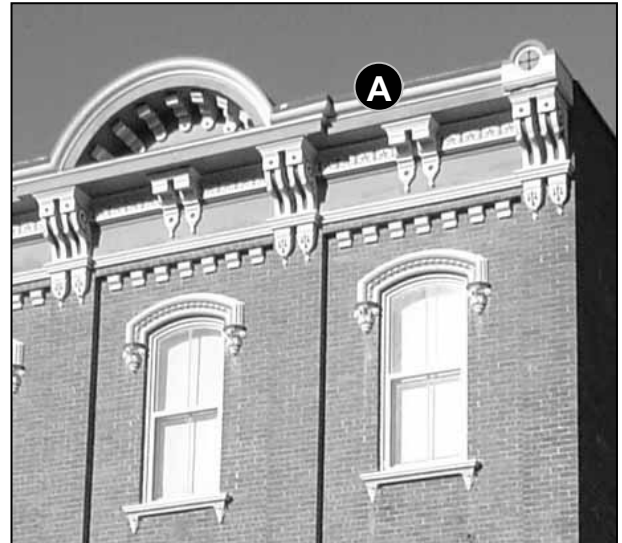
Fig. 5-77: 332 Main St. Subtle uses of color add intricacy and added depth to the cornice of this building.
