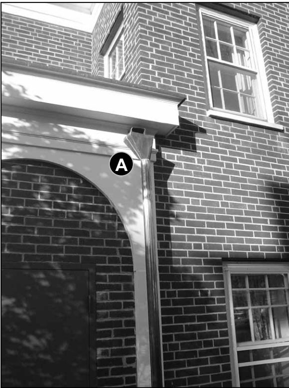
Fig. 5-54: 116 South St. A new copper downspout has been installed here to match the original materials.
