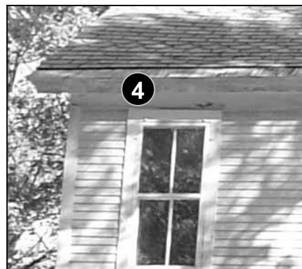
Fig. 5-55: 220 Silver St. The original copper eave flashing still remains along the edge of this roof.
