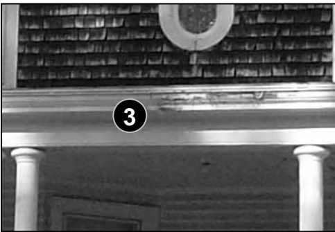
Fig. 5-53: 133 Elm St. The wood trim here is showing signs of moisture damage, and will get worse if left un-repaired.
