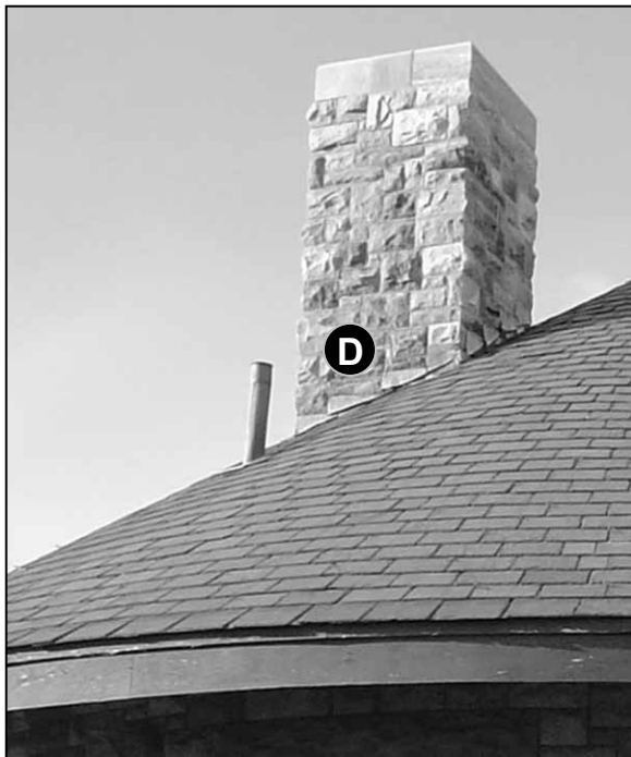
Fig. 5-50: 150 Depot St. The original soft-metal flashing along the bottom of this chimney remains in good condition, and has weathered to match the color of the stone.
